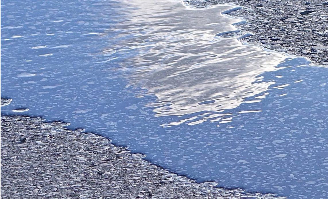
Water pooling on asphalt
